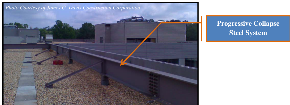
Figure 2 | Progressive Collapse System Installed
